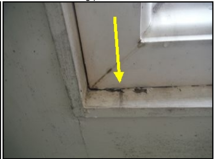
Soft fascia on front behind gutters.
