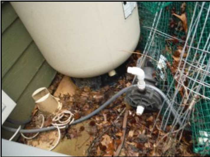
Suggest removing pool pump and filter. Pool has been filled in.
