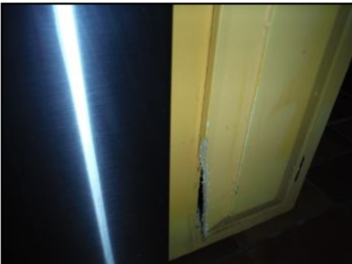
Damaged kitchen cabinet doors.
