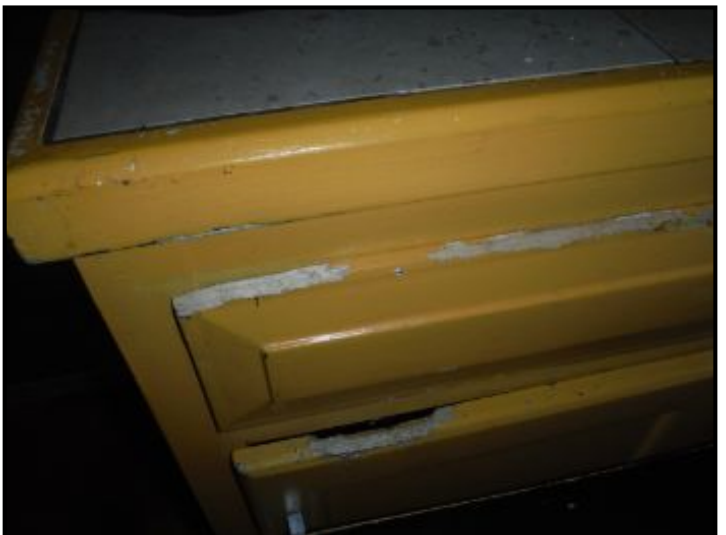
Damaged kitchen cabinet drawers.
