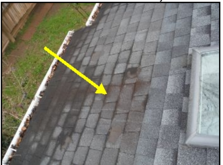
Rotted decking below master bath skylight.
