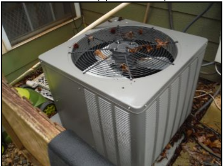
Condensing unit. Manufacture 2014
