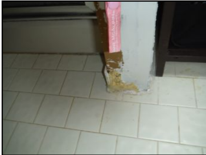
Missing baseboard tiles.
