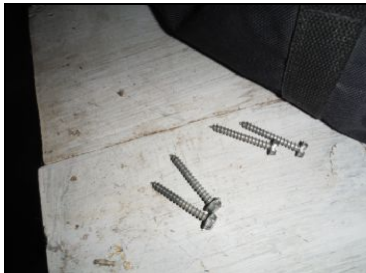
Panel cover screw should not have pointed ends. Can damage wiring.
