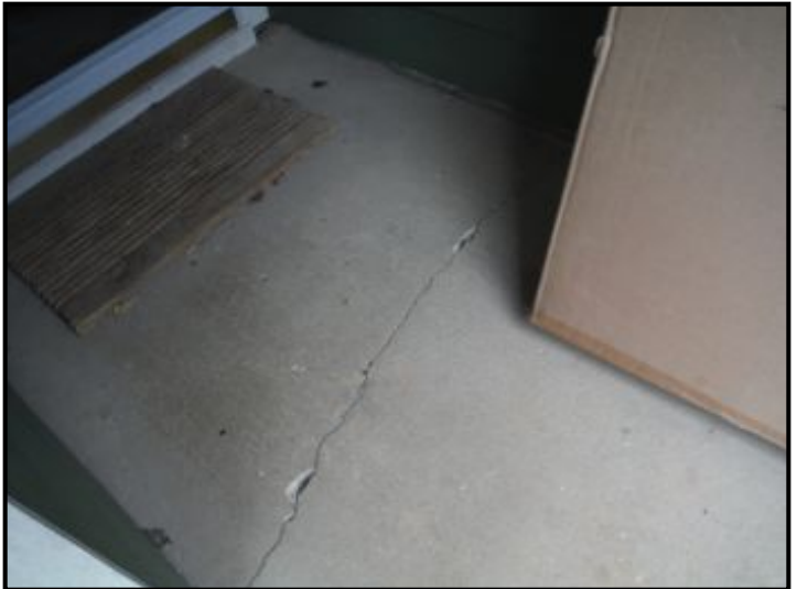
Cracks in side walk.
