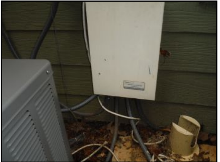
Suggest removing all electrical wiring for pool pump.
