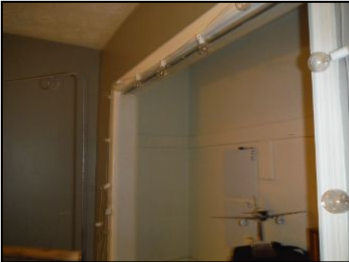
Missing closet door in rear bedroom.
