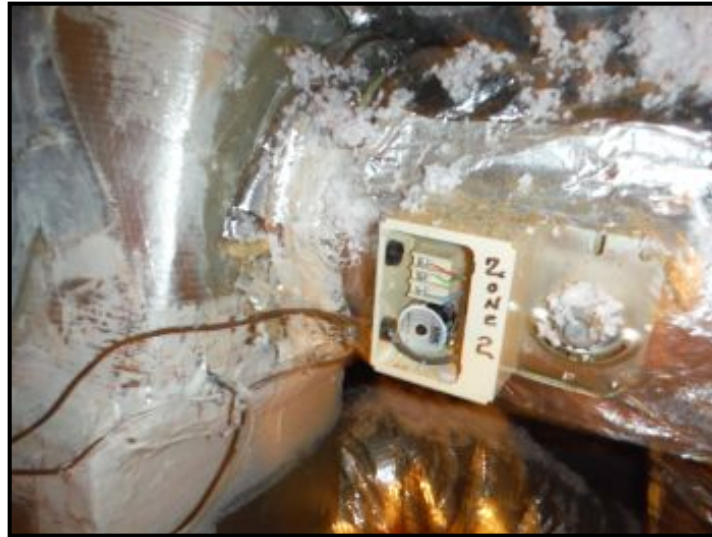
Damper system on ducts.
