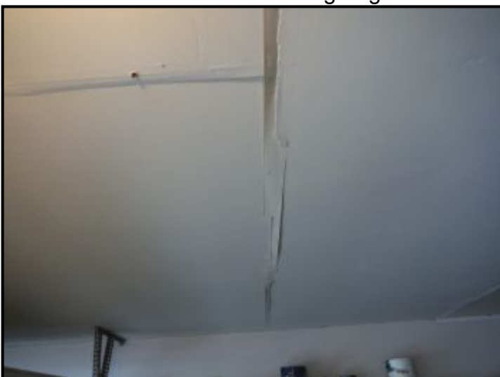
Ceiling tape coming loose in garage.
