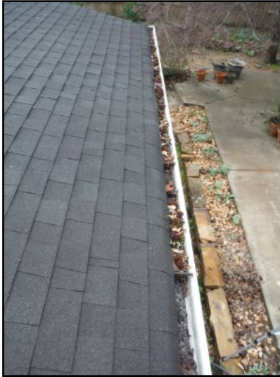
Gutter need cleaning.
