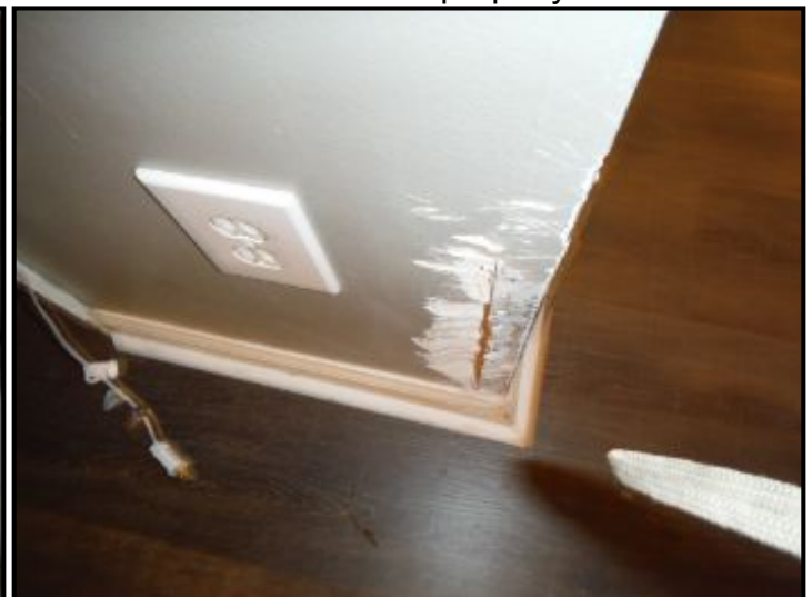
Damaged wall in rear bedroom.
