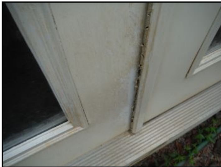
Damaged weather strip on side entry door.
