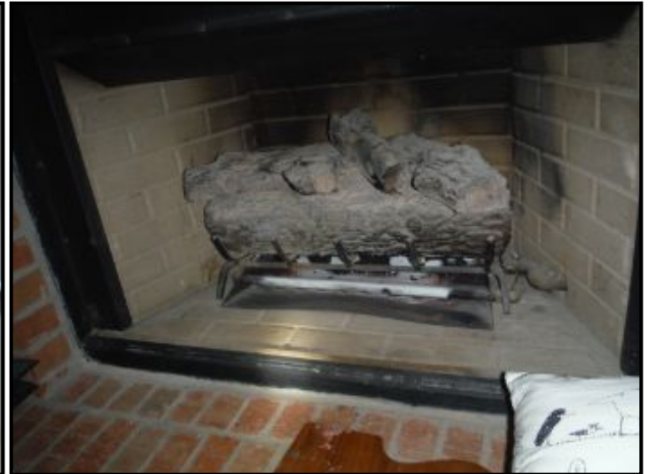
View of fireplace. Screen is missing.
