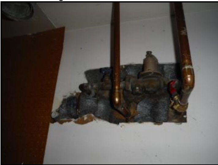
Main water shut off in garage.
