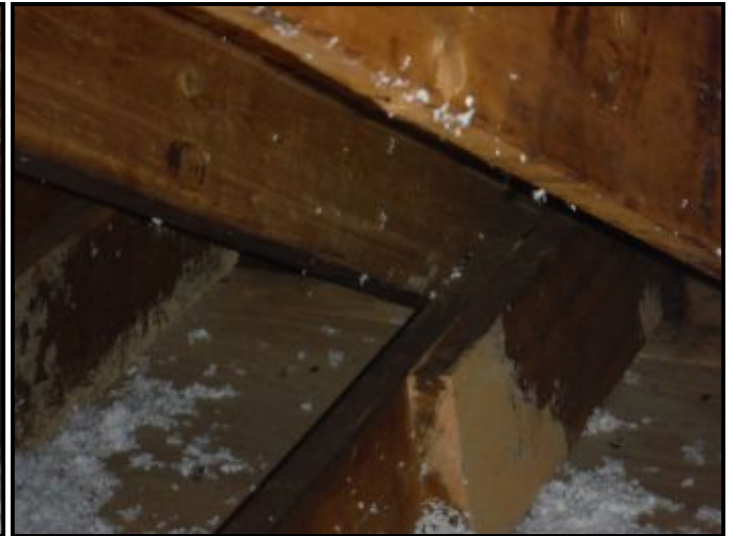
Missing insulation over kitchen.
