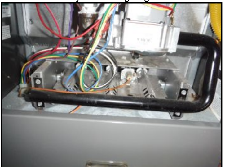
View of gas furnace.
