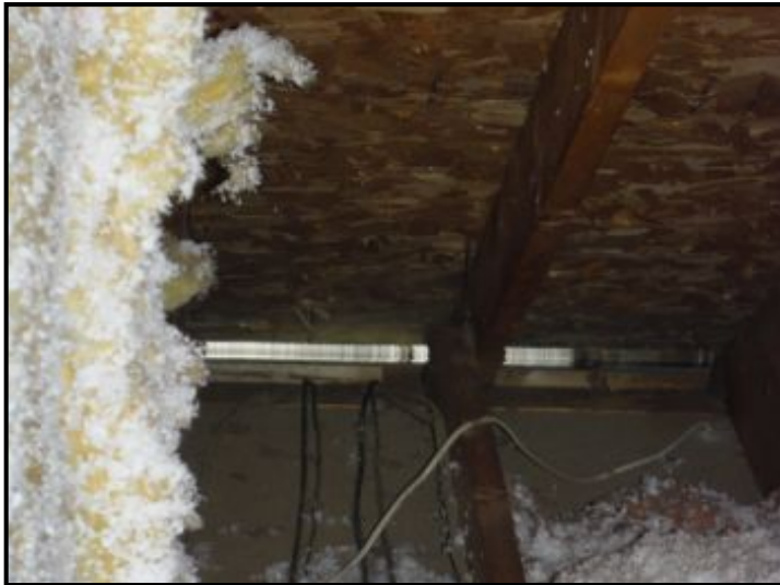
Missing insulation over kitchen. Replace.
