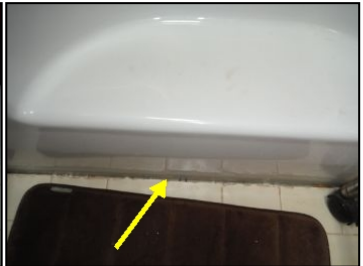
Missing tiles at garden tub.
