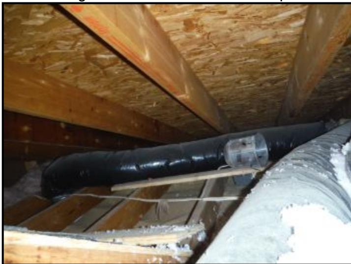
View of attic area over the porch addition. Insulation needed.
