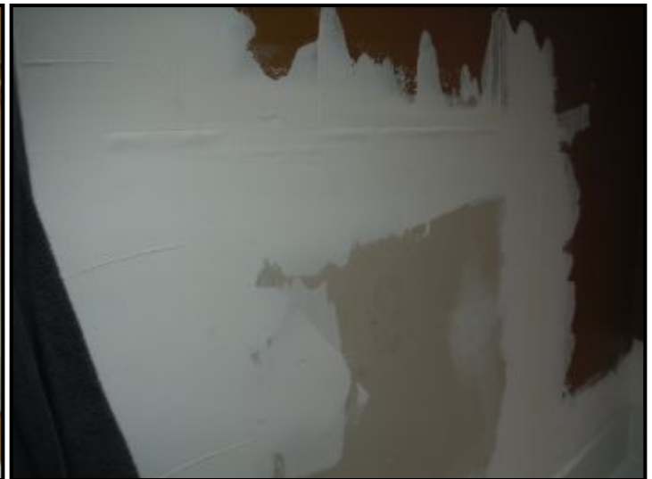
Walls in bath are not properly finished.
