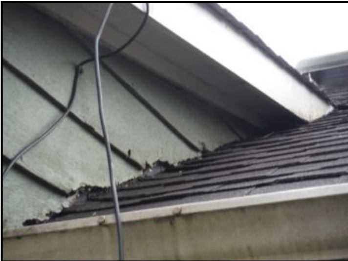
Damaged siding on rear porch addition.
