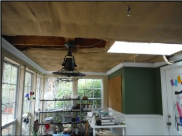
Ceiling to rear porch addition has been removed. Covered with cloth. Not able to visually inspect framing.
