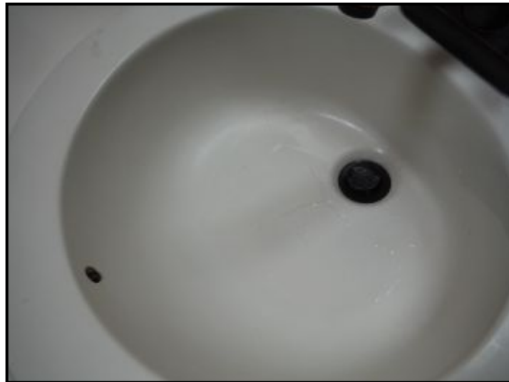
Cracked sink bowl.
