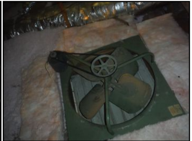
Attic fan. Not tested.
