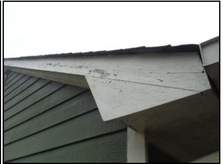
Peeling paint on fascia.
