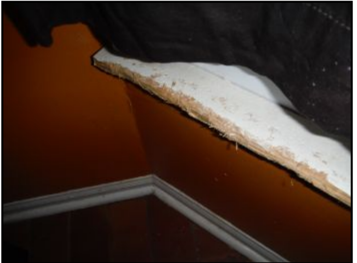
Damaged window trim in kitchen.
