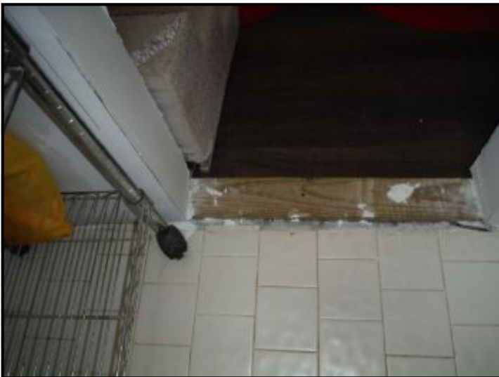
Unfinished tiles in door frames.
