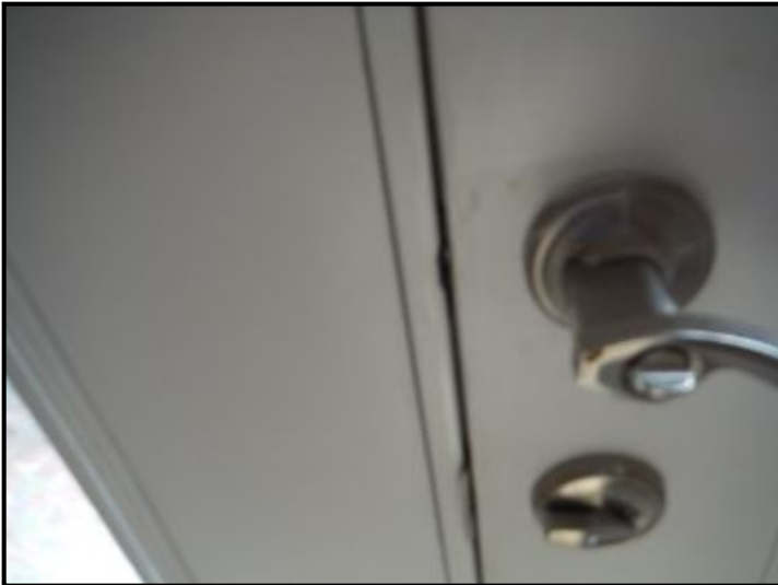
Door latch to side door does not catch. Adjust the strike plate.
