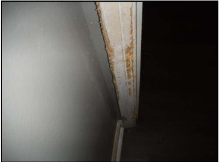
Damaged door molding in rear bedroom.
