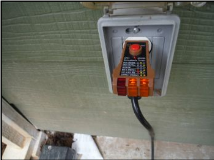
Exterior outlets should be GFCI protected.
